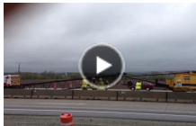
Crane topples over on U.S. 41 south of Scheu... Apr 20, 2012
